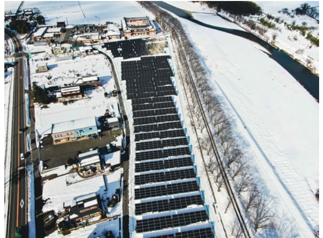
Solar power generation systems installed off-site at the Shiga Takatsuki Plant
